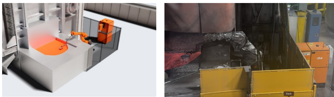
Figure 1. Automated sampling and chemical analysis system. Left: schematic illustration of a typical setup. Right: a system installed in a recycling plant.
